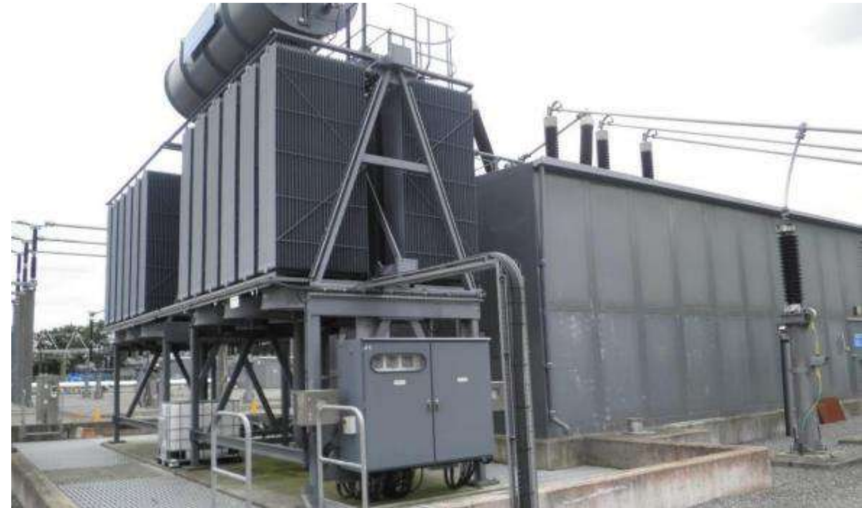
Typical 400kV Power Transformer
